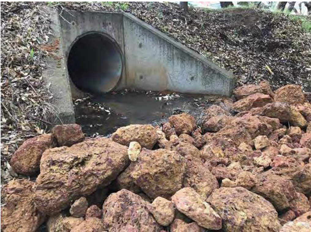
LEFT: The Pelham Brook modified outlet, with large rocks forming a riffle to slow the velocity, allowing the water to spread across the floodplain.
